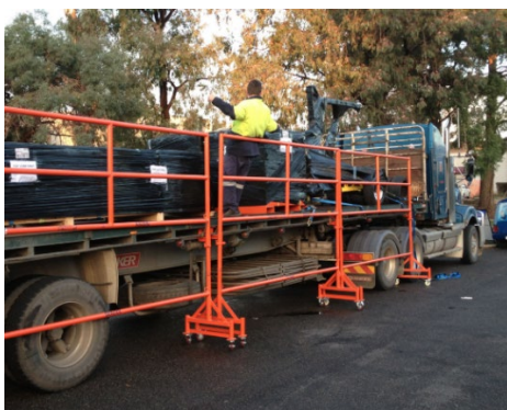
Edge protection system: BTS Flat Bed Trailer Edge Protection System (TEPS)
