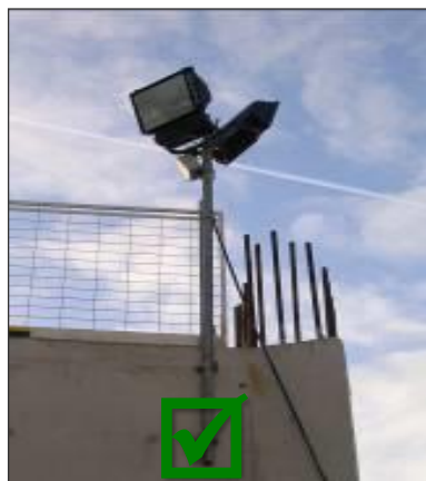
Halogen lighting in secure position easily and safely serviceable
